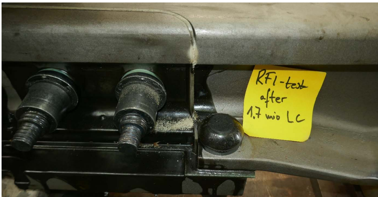
Figure 8: Opposite view of the butt joint after 1.7 million load cycles
